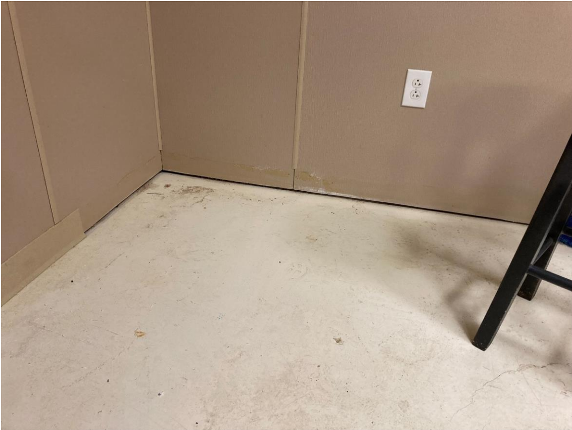
Updated pictures of concession stand damage as of 2/1/22
